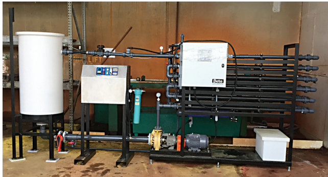
Fig. 6 — Pilot OxyFilter system.
